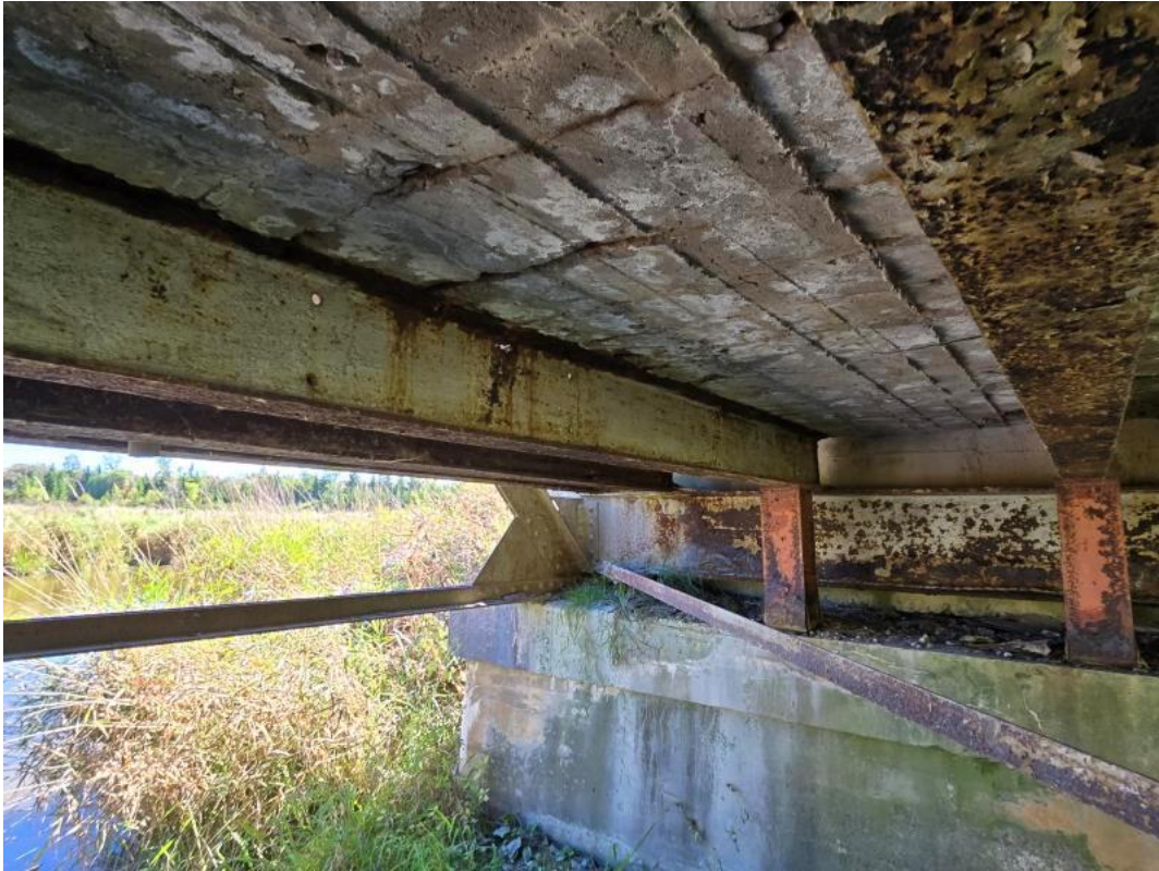
South Bay Corroded Perforated Web
