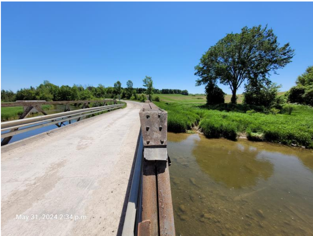
8-West Girder Slight Deflection
