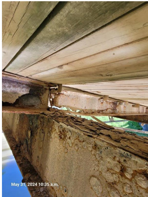
8-Crossbeam and Corroded Stringer
