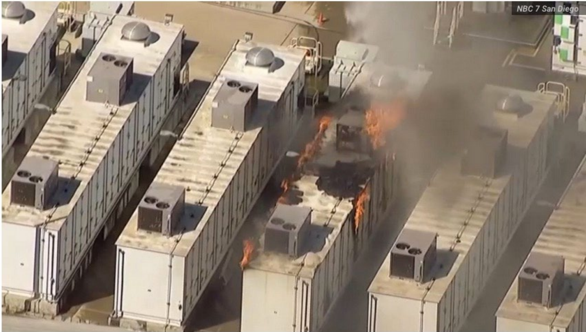
A fire burns at a SDG&E lithium-ion battery facility in Escondido, prompting evacuations, Sept. 5, 2024.
