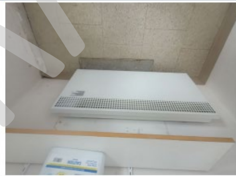
View of Newer Heater
