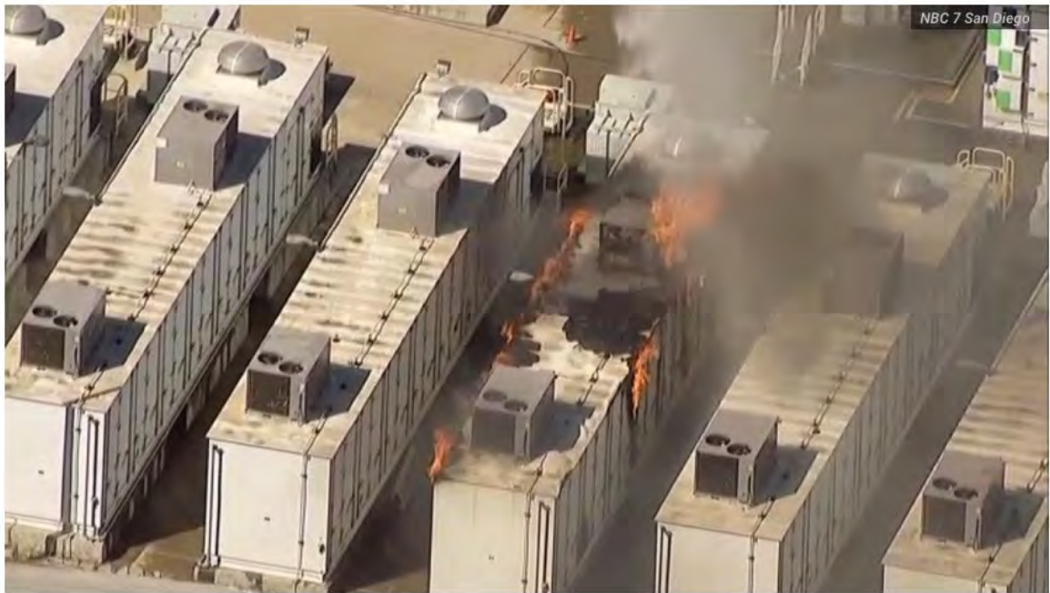
A fire burns at a SDG&E lithium-ion battery facility in Escondido, prompting evacuations, Sept. 5, 2024.
